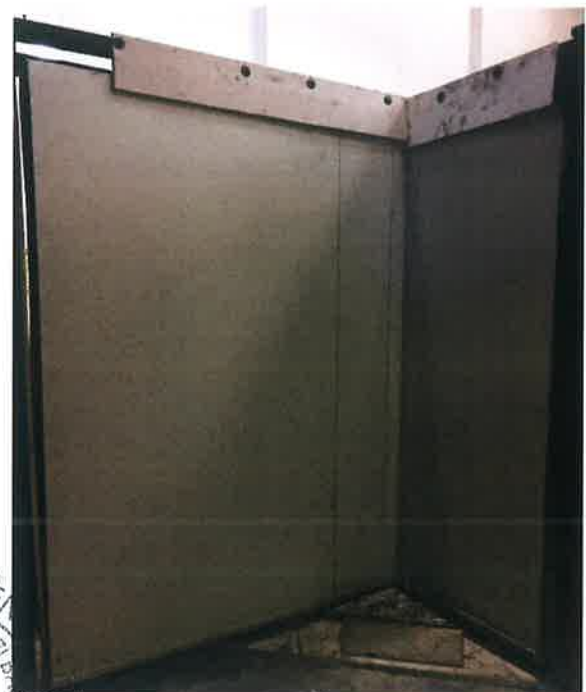
Photograph 6. Corner detail of Sample 1
